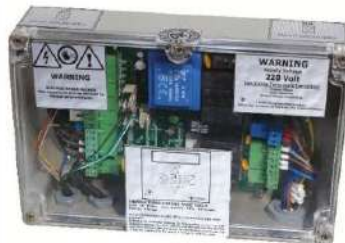
Internal control unit
